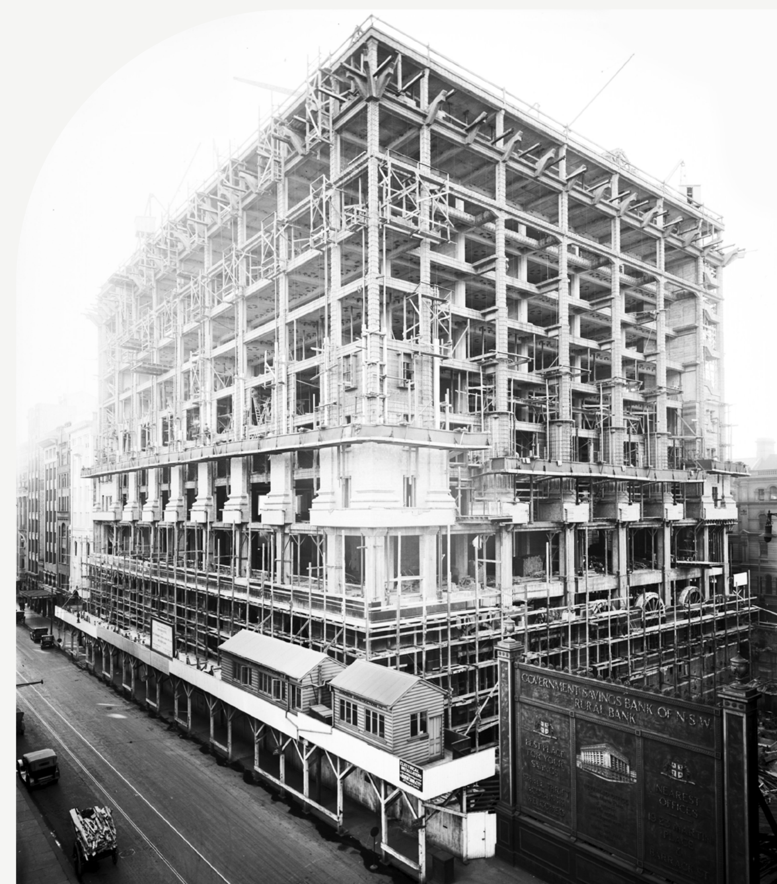
The construction of 50 Martin Place by the Government Savings Bank of NSW, 1926
